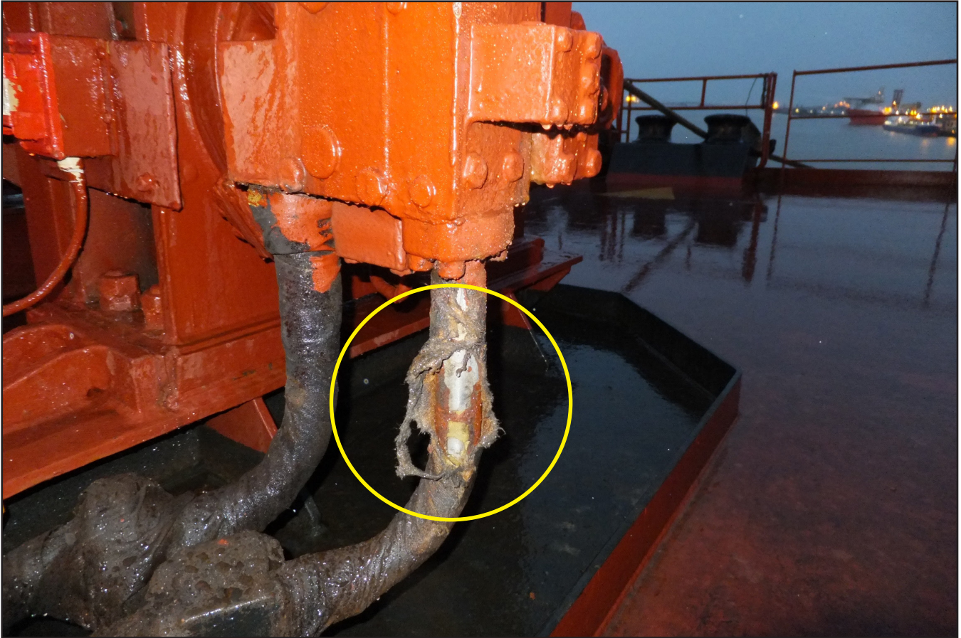
Figure 3: Chaffing marks on hydraulic pipe of starboard winch
